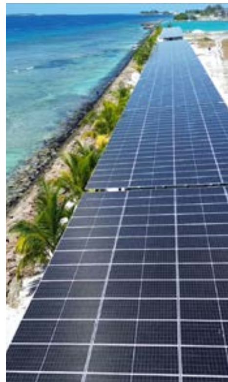
Solar power Location: Feydhoo Harbour, Maldives
