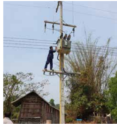
Transmission line construction project at Nong Ping village, Pathoumphone district, Champasak province.
