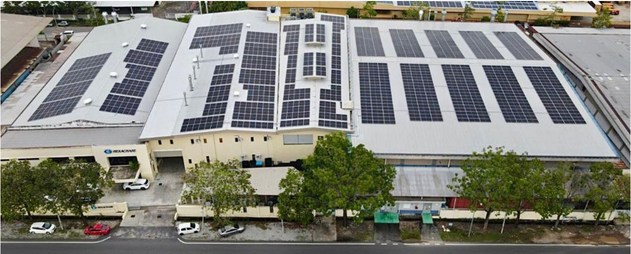
0.65 MW Solar Installation at Hexachase Flexipack, Malacca.
