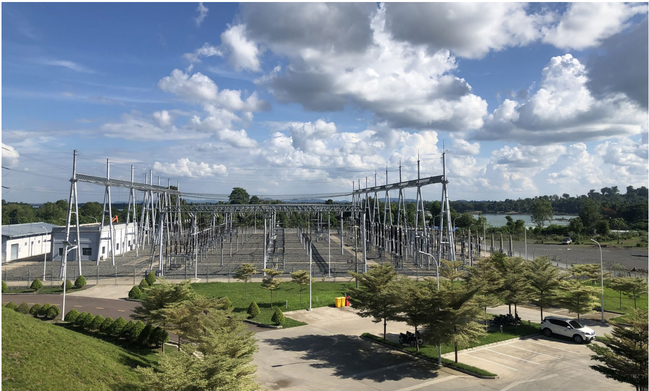
Transmissions lines connected to our 260MW hydropower plant at DSPC, Lao PDR.
