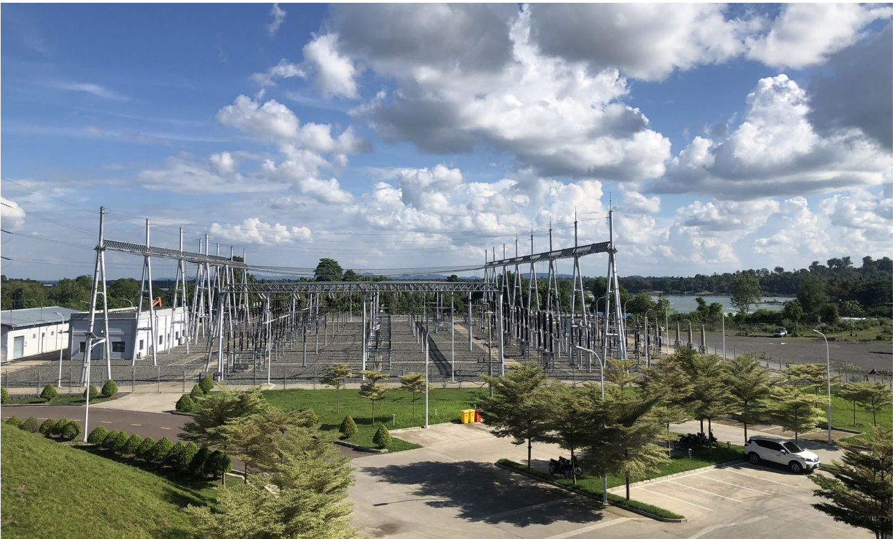
Transmissions lines connected to our 260MW hydropower plant at DSPC, Lao PDR.
