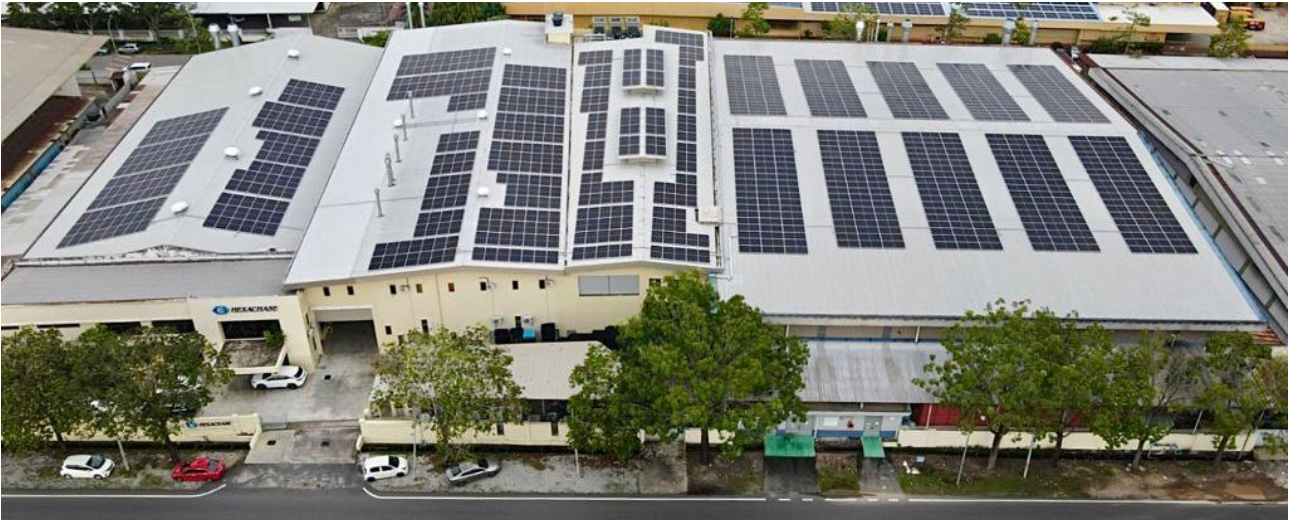
0.65 MW Solar Installation at Hexachase Flexipack, Malacca.
